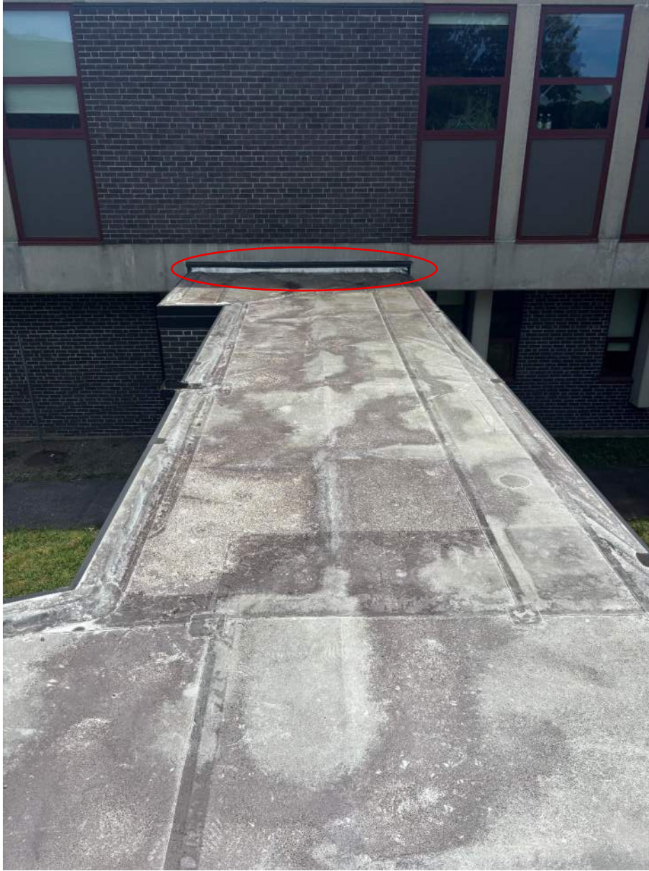
The curb (side wall) (circled in red) has a tar (vapor barrier) that is positive for ACM.
