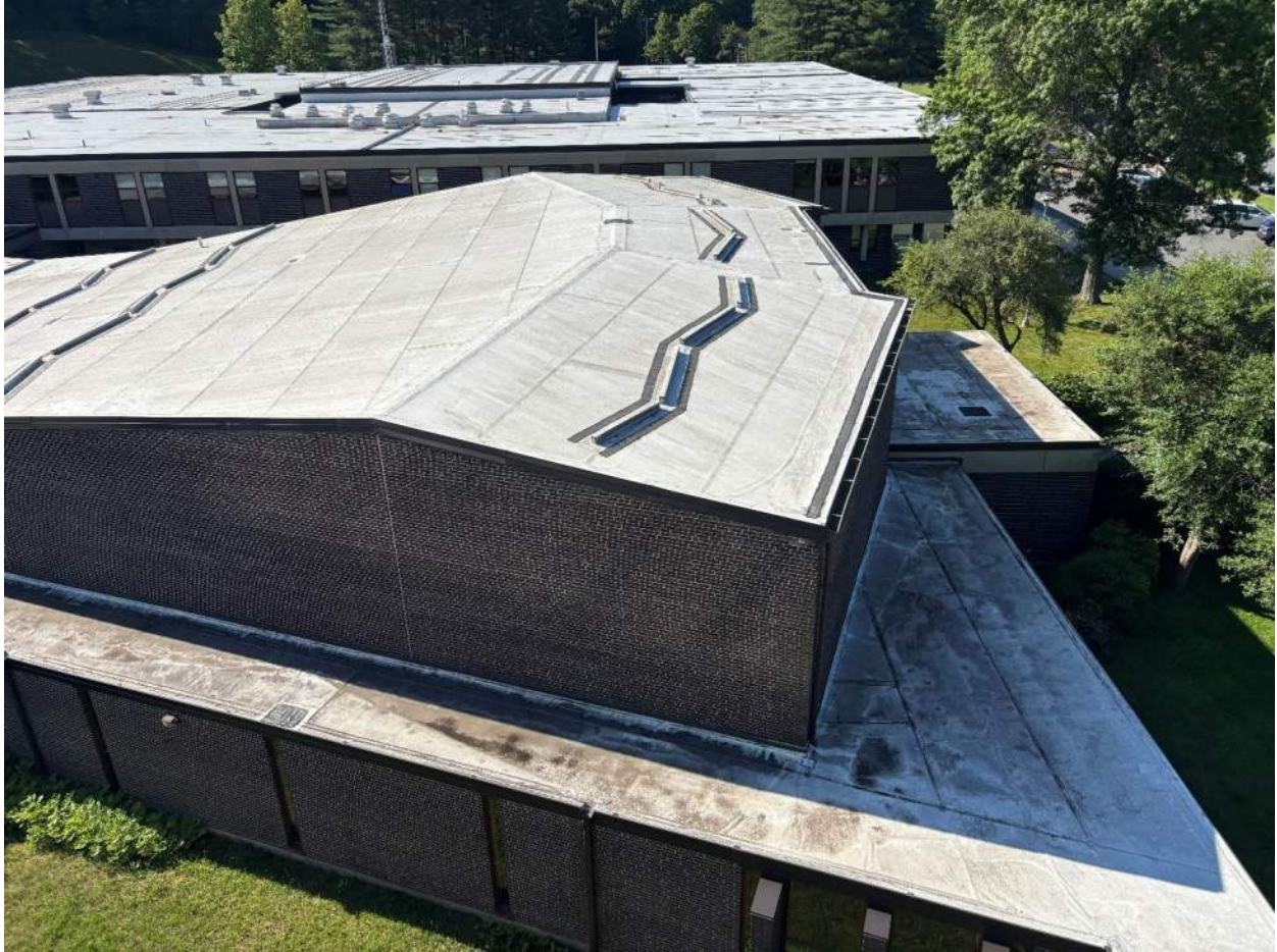
The gutter shown in this photo contains a Gray Sealant that is positive for ACM. (Gutters on either end of the auditorium roof)
