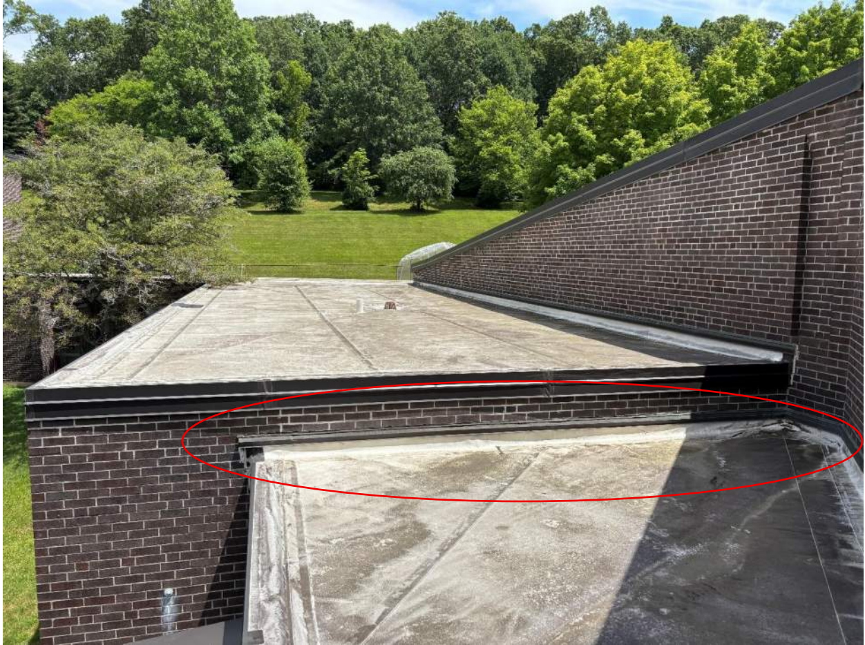
The curb (side wall) (circled in red) has a tar (vapor barrier) that is positive for ACM.
